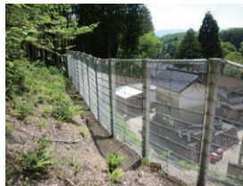
崩壊土砂防止柵 (HEF工法、HR-010009-VE ★)
